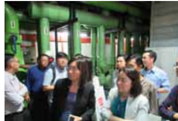
The TTT included a visit to the CoGen plant
